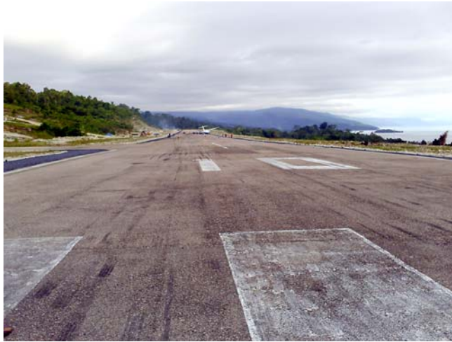
Figure 2: Area of no wheel marks from PK-TXL on the runway
